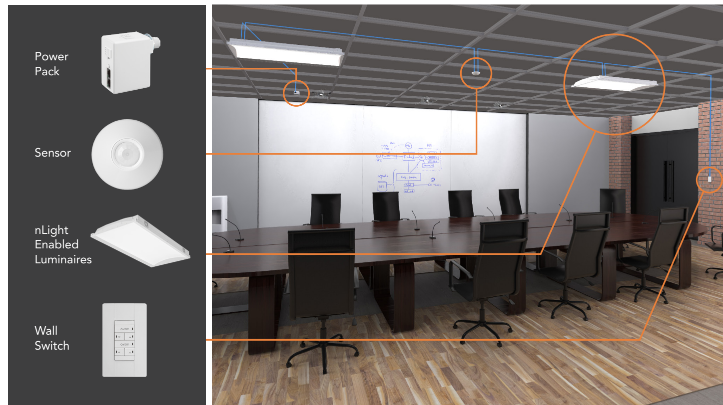
Example with nLight Enabled Luminaires
